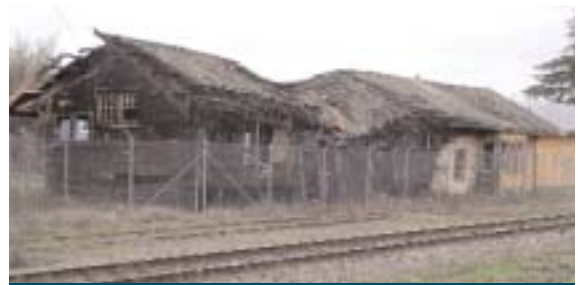
Novato Depot in disrepair
